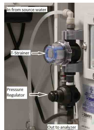
Figure 13 - Pressure regulator and T-strainer
